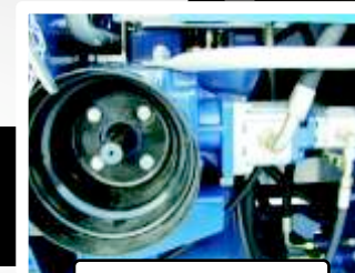
Two oil pumps
